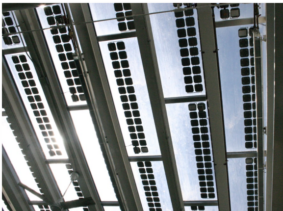
A building integrated solar photovoltaic (BIPV) system installed in the skylights at the Marjorie McNeely Conservatory at Como Park in St. Paul, Minnesota.
