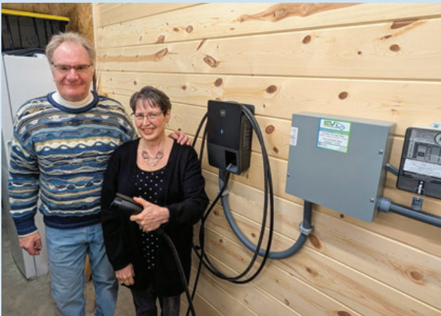
The Paviks installed a GM-provided Level 2 EV charger in their garage on BEC's off-peak program.
